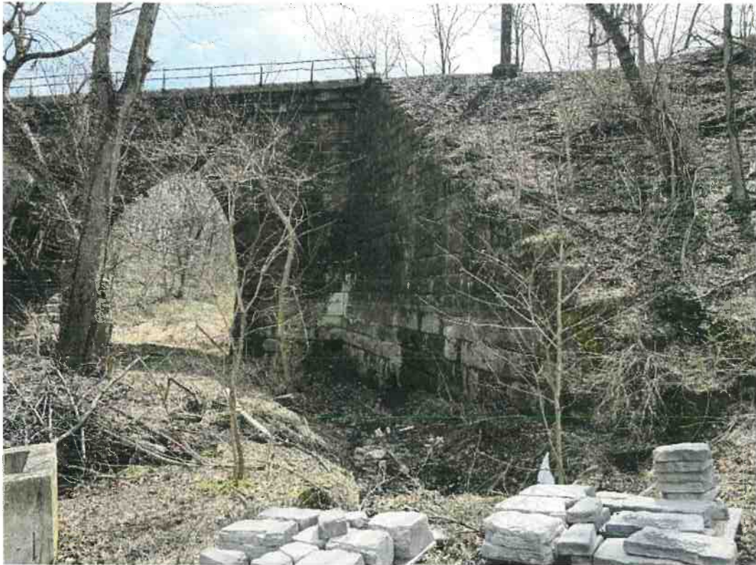
Photograph 5 – Disturbance near the west wingwall and abutment, facing southwest.
